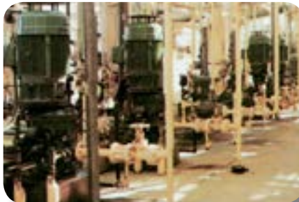
▲ 40 HP LMV-322 reactor feed pumps in a gulf coast refinery.
