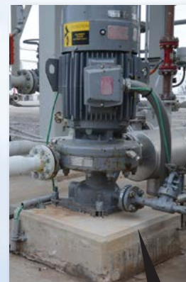
Sundyne Pump (Deethanizer Booster)
